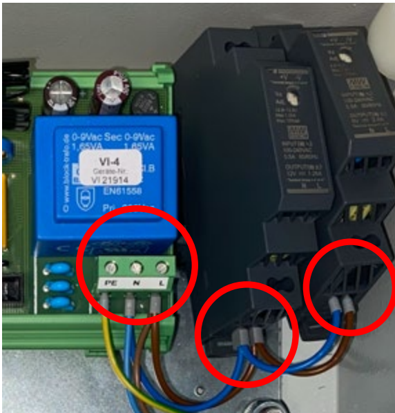
Figure 17: Power supply cabling
