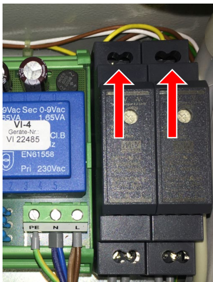
Figure 16: Power supply units, cabling
